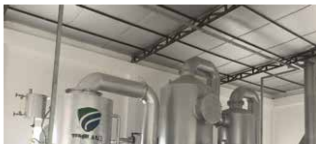
Incinerator in our plant
